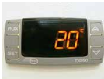
Air-conditioned electrical cabinet
